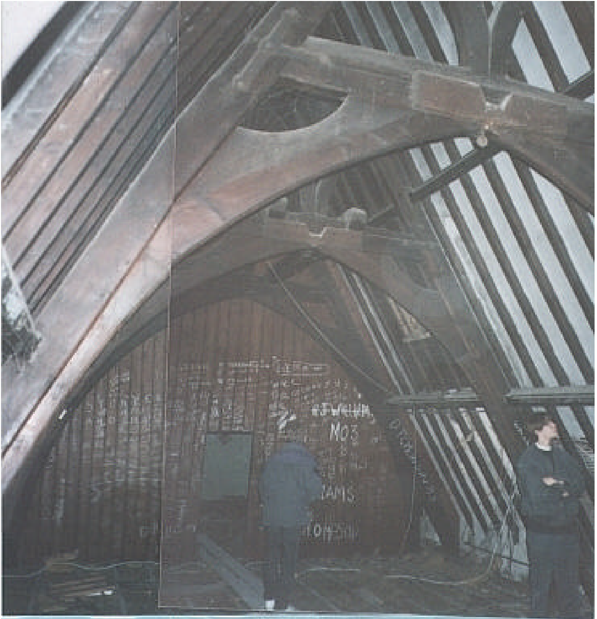
This is the east end of the roof space above the old “Big School” The bell rope can still be seen in the corner of the picture.
